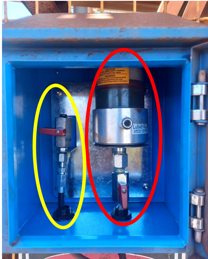
Accumulator Monitoring box containing accumulator with ball valve (circled red) & return line with ball valve (circled yellow)
